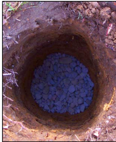
Figure 6 - Adding Gravel to the Bottom of the Hole is Not Required, but Can Be Beneficial
